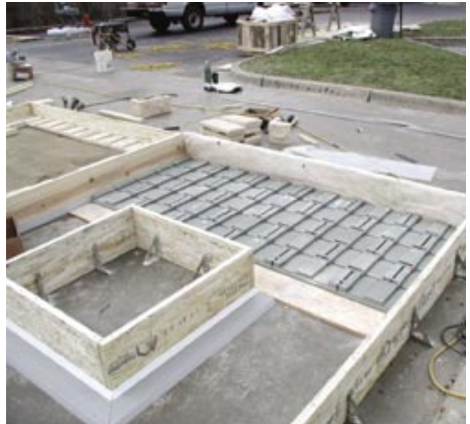
This sample panel, used at a construction demonstration organized by CON/STEEL Tilt-Up Systems, illustrates the Chameleon Wall System's ease of installation, even around panel openings
