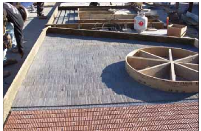
Shake form liner and Brick Snaps are placed in the form, ready for concrete.
