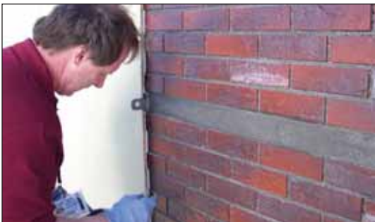
Upon removal of the vertical forms, the real brick finish is revealed. A strip of flagstone texture is used to conceal ties and is easily patched once forms are stripped.
