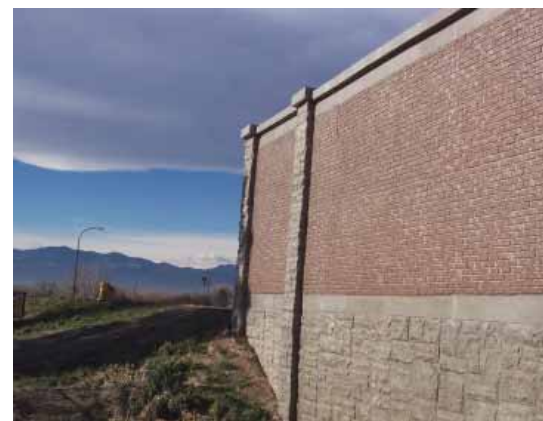
Poured-in-place concrete wall is adorned with Rough Brick and Ashlar Stone patterns on this residential community wall in Arvada, CO
