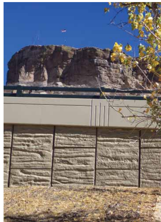
Front Street Flyover in Castle Rock, CO features a custom, rugged stone texture.
