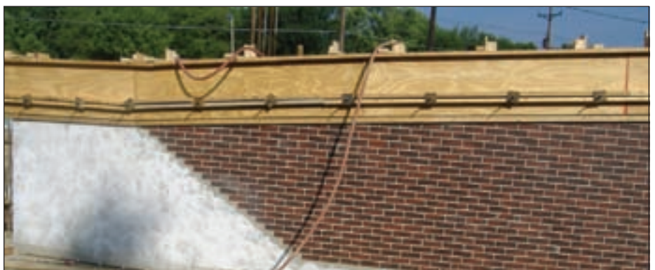
Vertical forms with Rim Snaps™ have been removed, exposing the brick façade finish.
